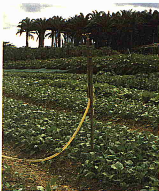
Overhead sprinkler system
